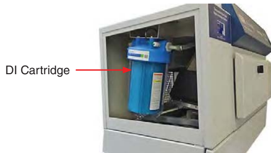
Figure 8d: Deionization enclosure access panel removed showing DI cartridge.
