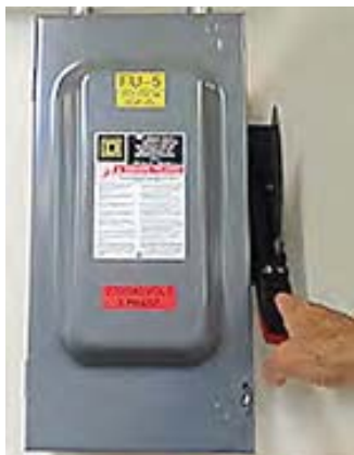
3. Main power OFF.
