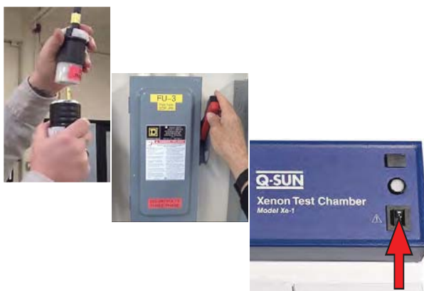
28. Reconnect Power. Power ON. Xe-1 power ON.
