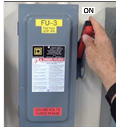
22. Main power ON.
