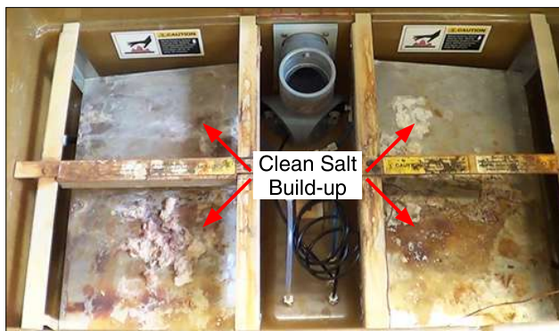
Figure 14.1c: Metal plate chamber heaters with salt build-up.
