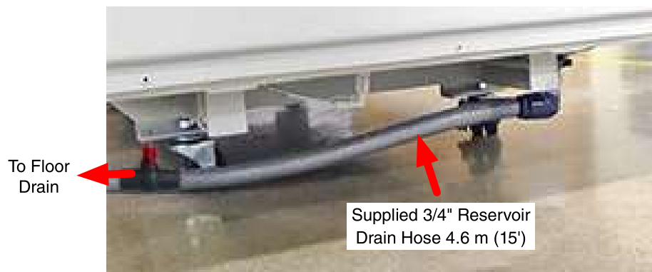
Figure 6.6e: Solution reservoir drain connection.
