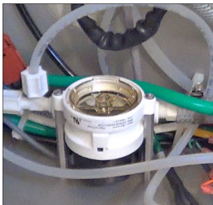
Figure 8.18c: Shower flow sensor.
