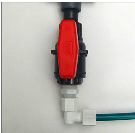
Figure 8.19b: Shut off valve open for ECC1 test.
